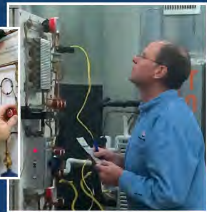
One of the Cochise College HVAC students learning trouble-shooting on the TU-100.
