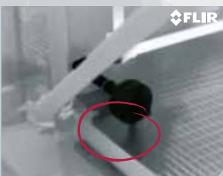
A leaking pressure gauge.
