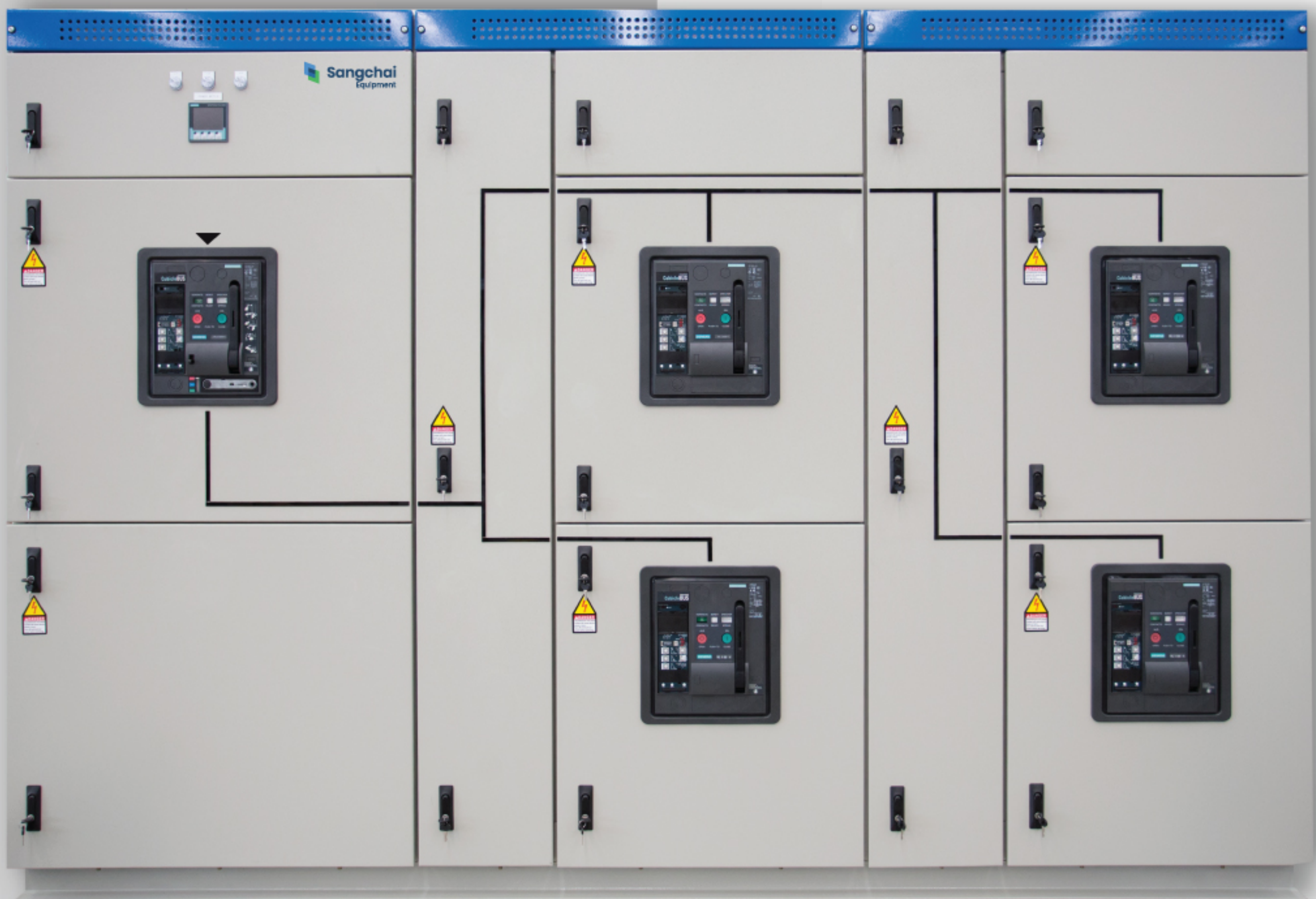
MDB : Main Distribution Board for design verification test
